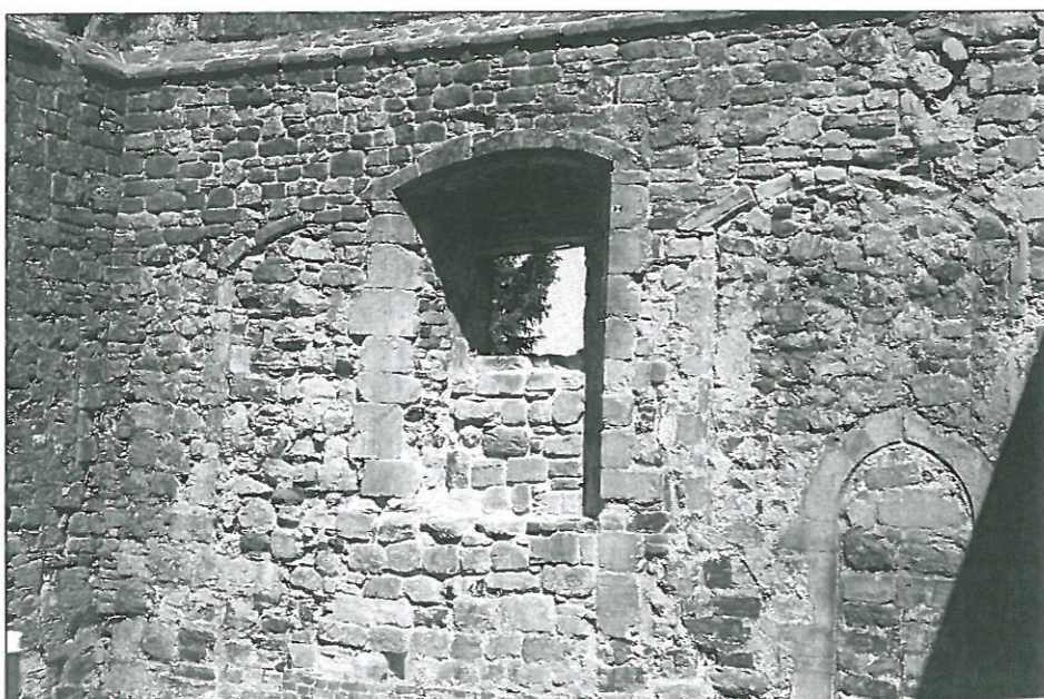
BELOW: The east wall of the courthouse, showing the different phases of building.
